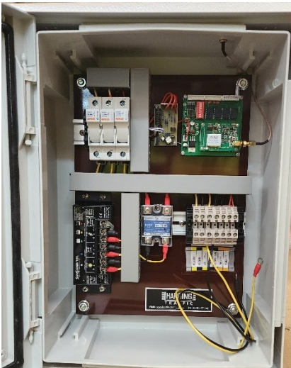
Sign activated via Loop Detector
